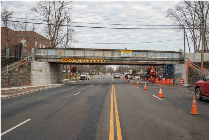
Looking north at the existing bridge over Cherry Valley Avenue in Garden City on the Hempstead Branch on March 1. Jeff Erlitz photo
