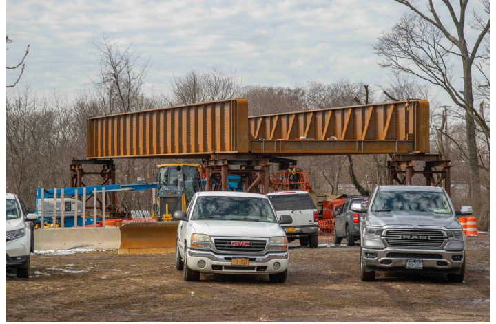
The new bridge has been assembled and is located just south of the right-of-way and just east of Cherry Valley Avenue. This is looking northwest. Jeff Erlitz photo
