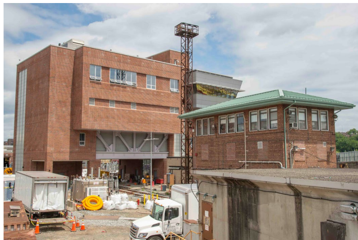
The old and the new. On the left is the new 207th Street Yard Master Tower, on the right, Tower A. This and all of the other photos were taken June 4.
