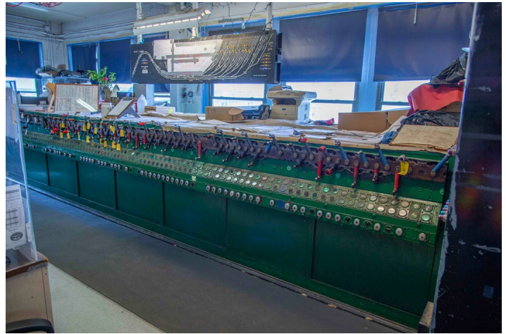
The 107-lever US&S Model 14 machine in Tower A. It was placed in service around 1931.
