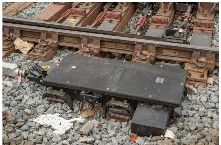
More traditional looking are the Twincos Model TMC-1 switch machines, which are mounted on either side of a switch, the usual standard practice.
