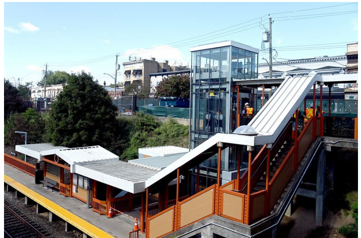
One of the new elevators at New Dorp on September 19. Marc A. Hermann/MTA photo
