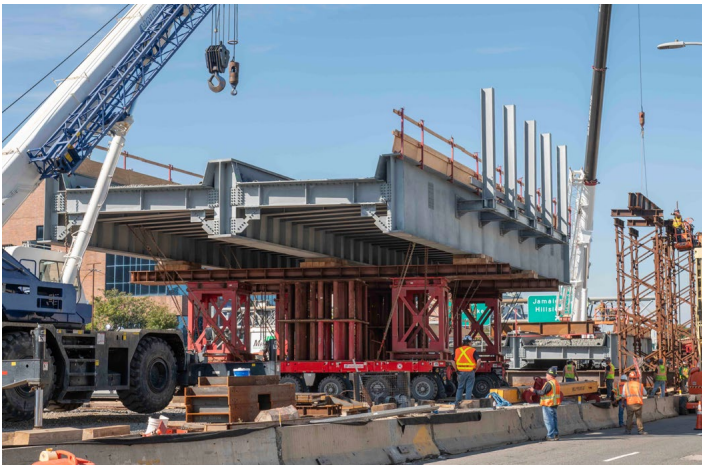
As was done last spring, the new bridge was assembled in the median between the expressway's northbound main and service roads.
