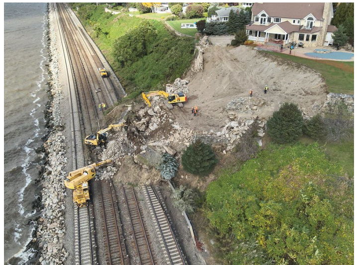
Aerial view of the Hudson Line landslide on October 22. MTA Police Department photo
