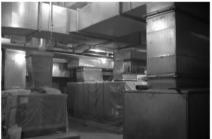
Second floor mechanical room.
