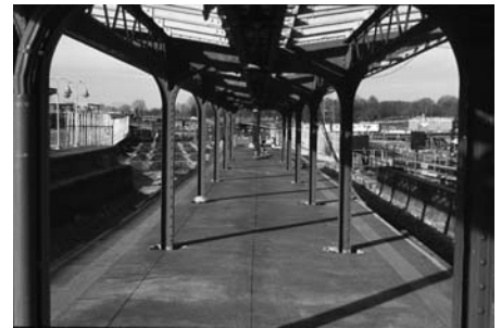
Atlantic Avenue platform, with view of Track K3/4, looking north, January 27, 2002. Jeffrey Erlitz photograph
