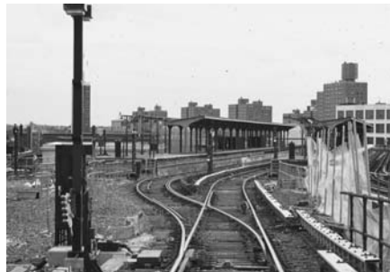
Switch #507, north of Atlantic Avenue on the Canarsie Line, August 5, 2001. Jeffrey Erlitz photograph
