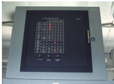
Another example of Mauell's work — 111 th Street Trouble Indication Panel on the Flushing Line.
