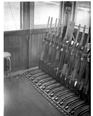
Interlocking machine in Bronx Park Tower, June 17, 1951.
