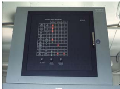
Another example of Mauell's work — 111 th Street Trouble Indication Panel on the Flushing Line.
