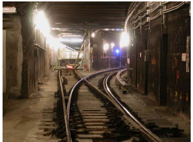
View north of new switch #187 south of the Canal Street station on the Nassau Street Line. Current northbound J trains diverge to the right. Later this year, northbound trains will proceed straight into the station on what is now the southbound express track.
