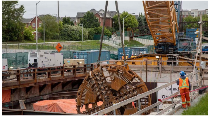
After being disassembled, parts of the TBM are carefully lifted out of the extraction shaft with a crane. Metrolinx photo
