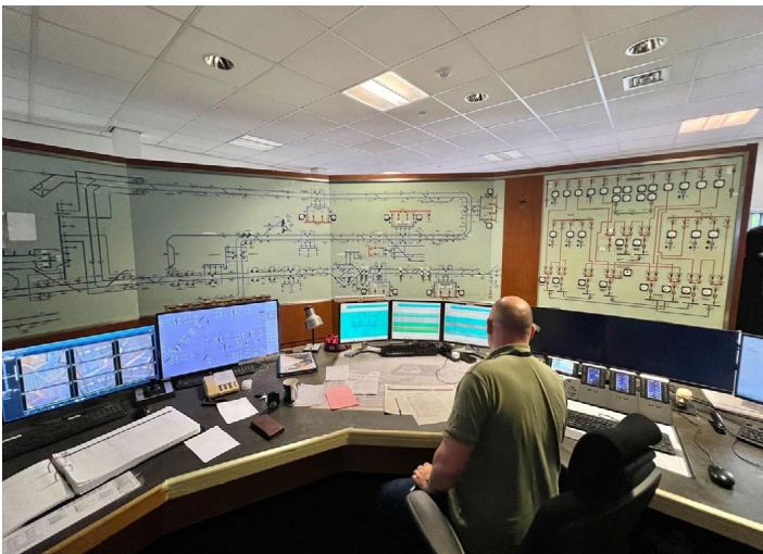
View of the current SCADA system at Tyne and Wear. Nexus photo
