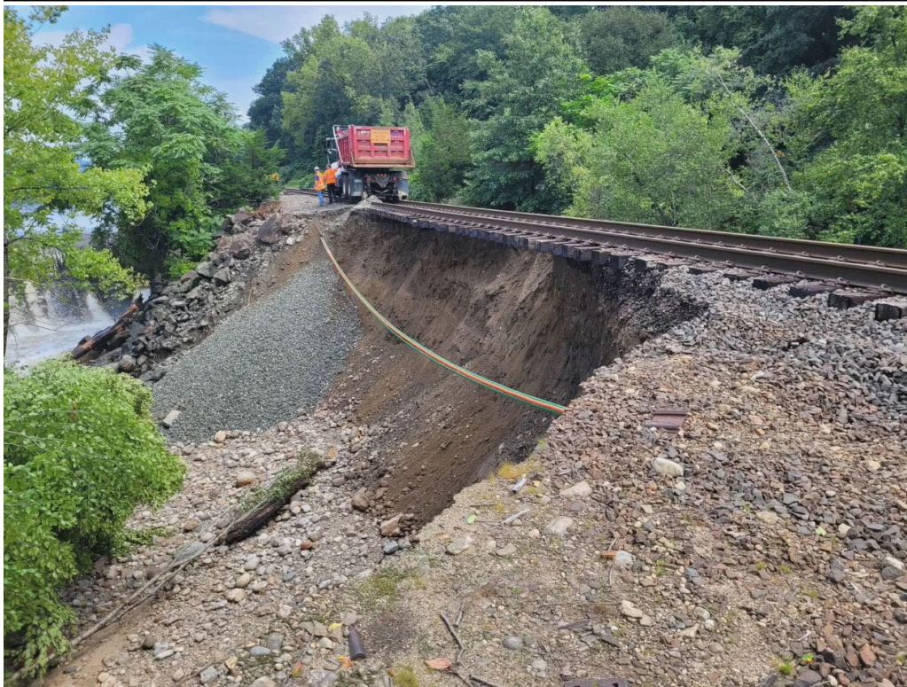
The washout between Seymour and Ansonia. Metro-North photo
