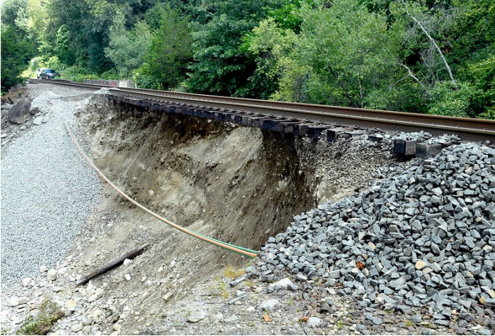
The washout, near Seymour, as seen back on August 22. Marc A. Hermann/MTA photo
