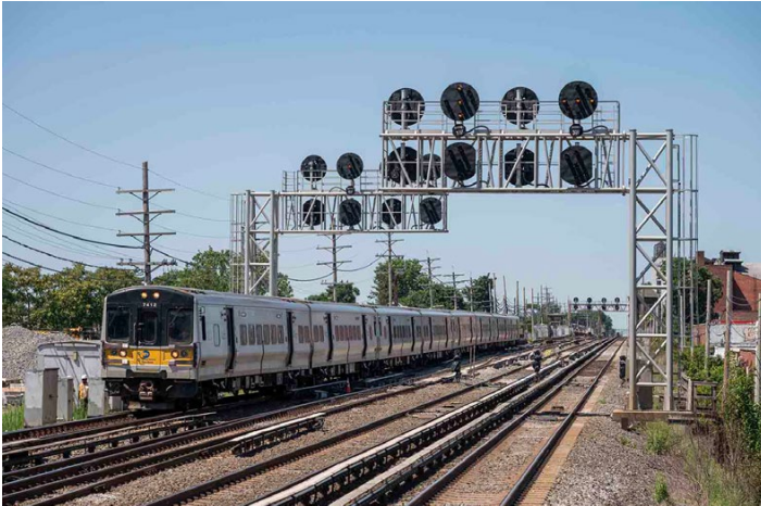
On July 23, two days before the signal cutover, Train No. 722 (Grand Central-Hempstead) passes under and by Signal Bridges No. 2, complete with eight traditional position light signals. M7 No. 7412 (Bombardier Transportation, 4/2005) is in the lead. The view is west from Elmont-UBS Arena Station. Jeff Erlitz photo
