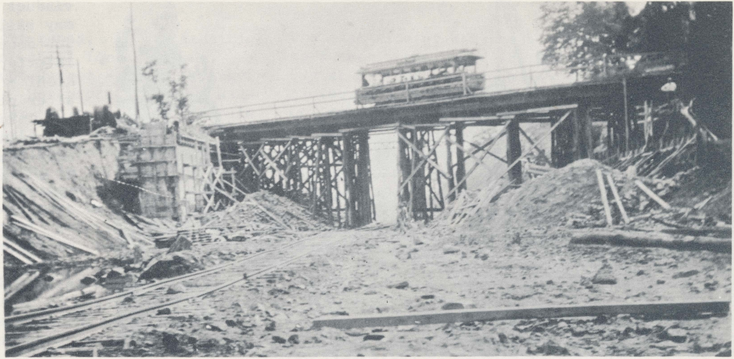
RIGHT - An open car of the W.E.R.R. crosses over the temporary bridge spanning the site of the yet-to-built Wykagyl Station (J.Tolley)
